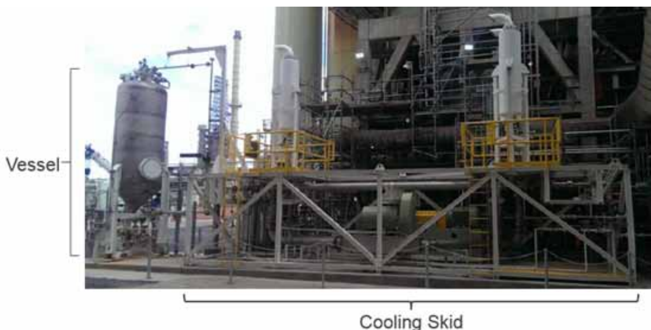
Image 1 – Continuous Catalyst Withdrawal (Mark-I) Installation – Marathon, Garyville 2
