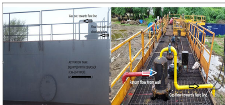
Figure 3: Installed Tank-Degasser Assembly
